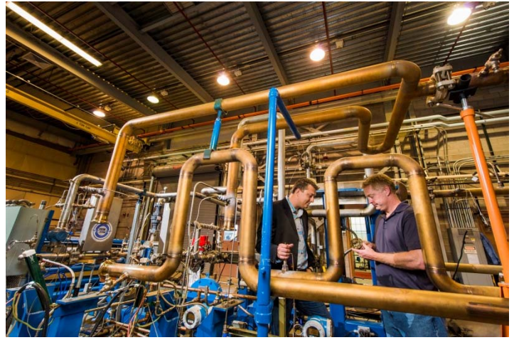
Jim Pasch, principle investigator of the S-CO 2 Brayton Cycle Research and Development Program, and Darryn Fleming, principal investigator of the S-CO 2 Brayton Heat Exchange Program, investigate a turbine and compressor inside a test facility at Sandia National Laboratories. (Photo by Randy Montoya)
